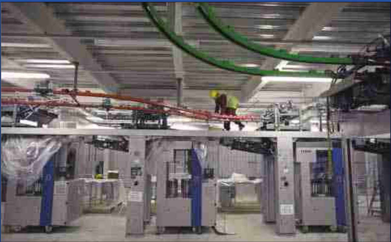
The new press installation at the Guardian Print Centre in London
